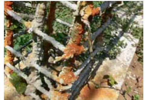
Iron rebar disintegrating and rusting
